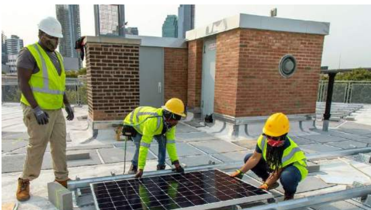
Image 8. Workforce trainees install solar on affordable housing development in Queens, NY. Photo credit: Sunwealth.
