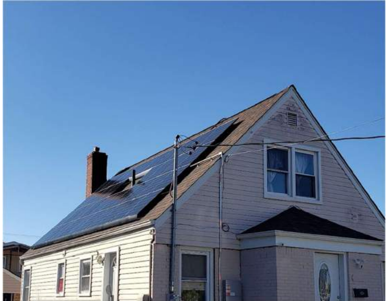
Image 19. Rooftop solar installation. Photo credit: 718 Solar.
