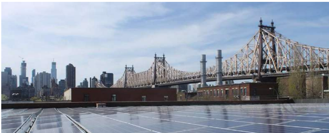
Image 1. Solar installation in front of Queensboro Bridge in New York City. Photo credit: NYSERDA.
