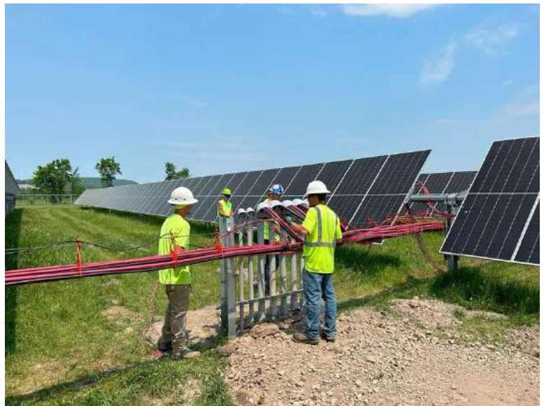
Image 2. Electricians completing wire management for an Upstate community solar installation. Photo Credit: GreenSpark Solar.
