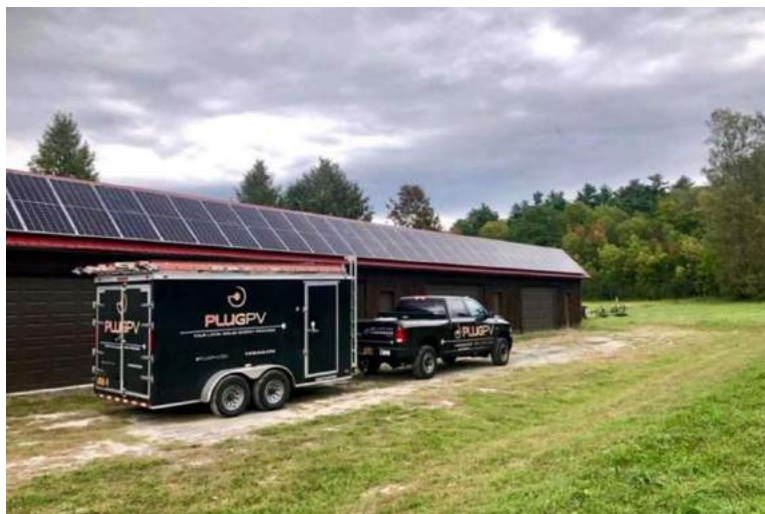
Image 19. Solar installation on a rural garage. Photo credit: PlugPV.
